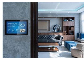
Smart building - Domotique
